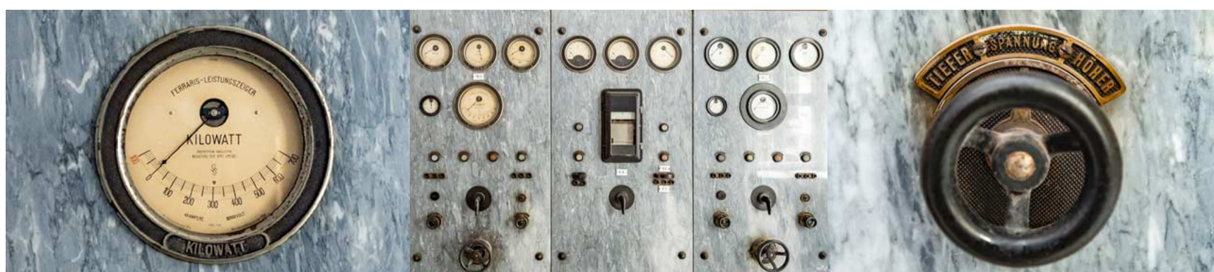
Photos below f.l.t.r.: Power meter, control elements, voltage adjuster for remote transmission at a depth of 272 metres
